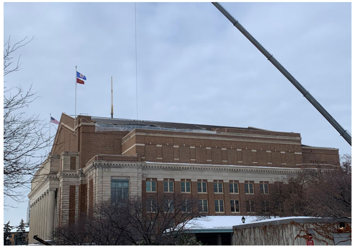
View of East Parapet Damage
