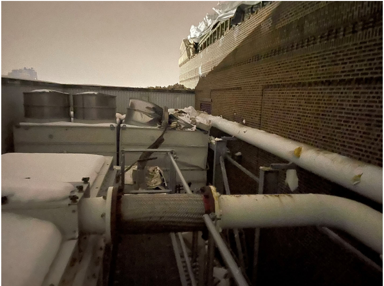
View of East Parapet Damage
